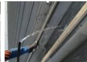
Roof cooling during the summer
