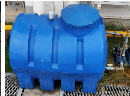
Air conditioning condensate water recycling system in Vietnam Plant.
